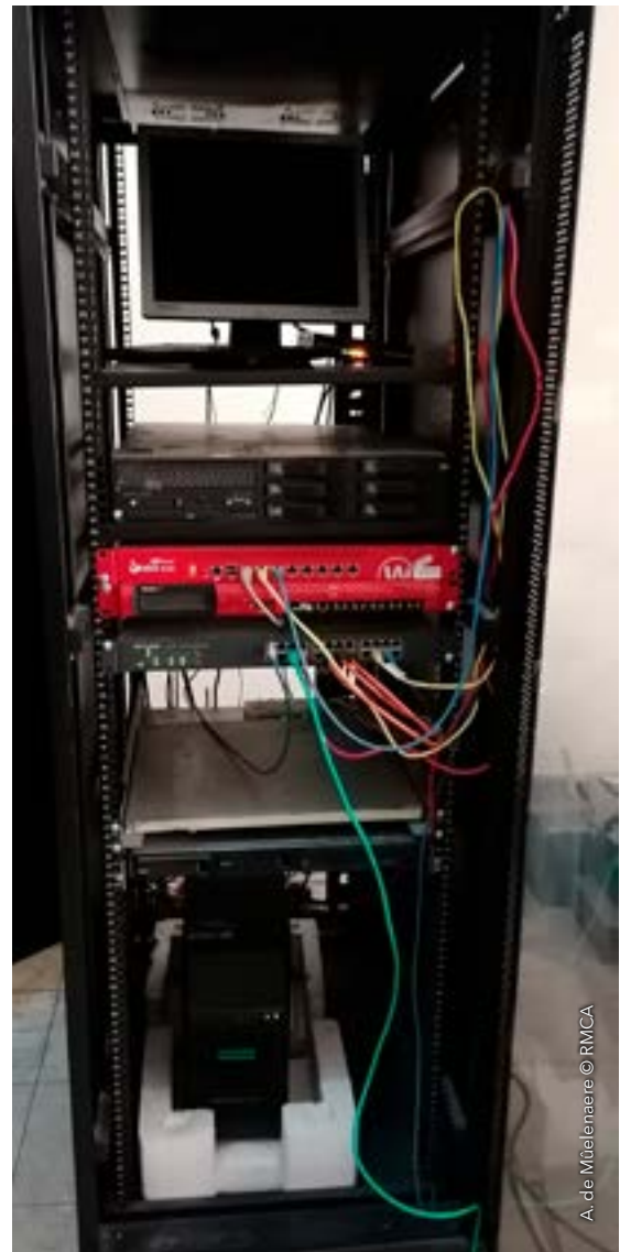
Mirror sites for the GeoRes4Dev project can be hosted at the CRGM thanks to equipment installed by the ICT service.
